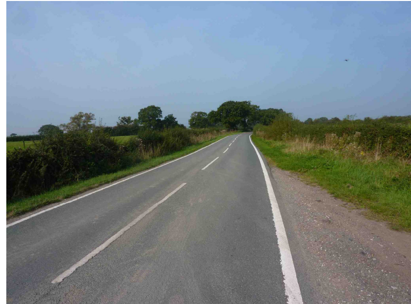
Figure 2 Inappropriate Line Markings
